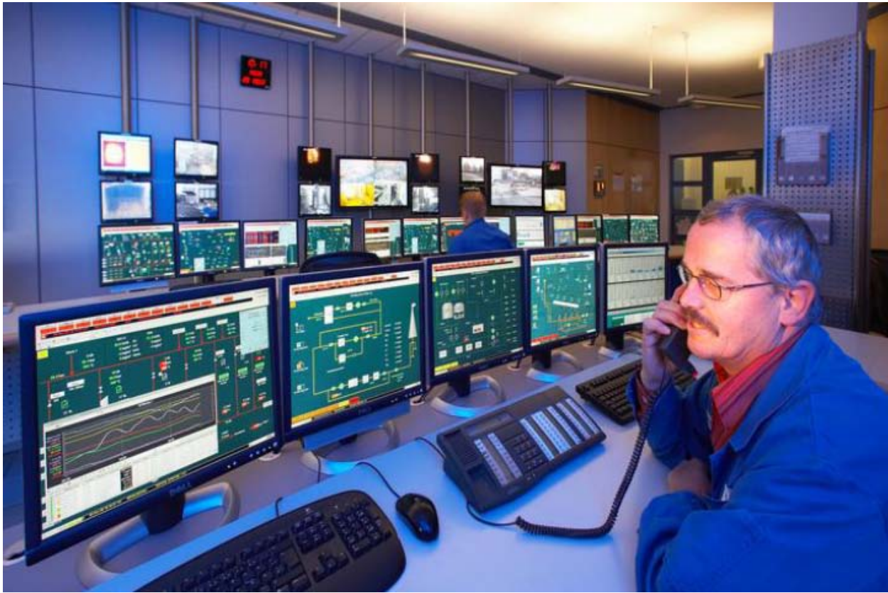
Figure 1. Alarm management in a process control application. The area on top of the screens in front of the operator show red blocks indicating alarms and part of the alarm list.
